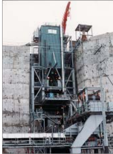
Fig. 3: Semi-mobile crushing plant Abb. 3: Semi-mobile Brechanlage
