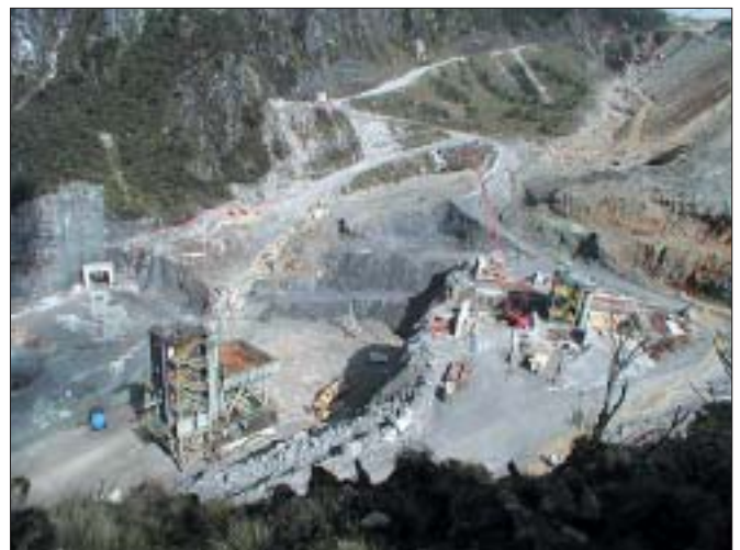
Fig. 7: One crushing plant approaching the "new pocket" with the other already in the new position Abb. 7: Gemeinsamer neuer Standort für beide semi-mobilen Brechanlagen
