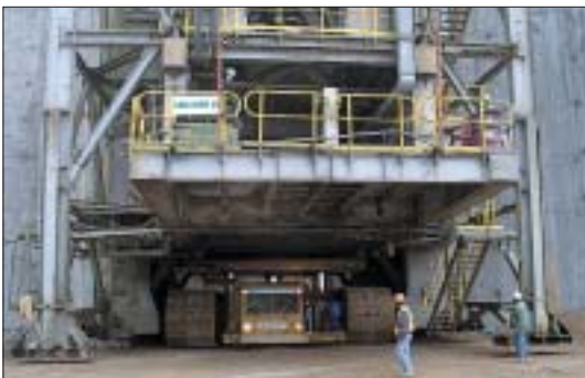
Lifting of crushing plant by transport crawler Anheben der Brechanlage durch die Transportraupe
